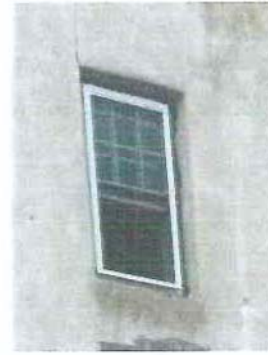
Unacceptable Window Usage
